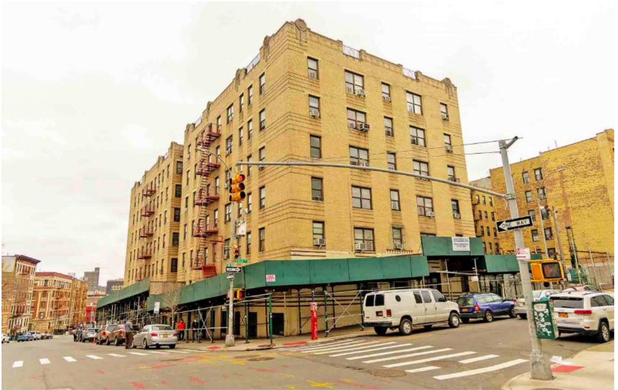
Mold grew dark on the bedroom walls at Tiebout Avenue, fed by faulty plumbing and a leaky roof.
